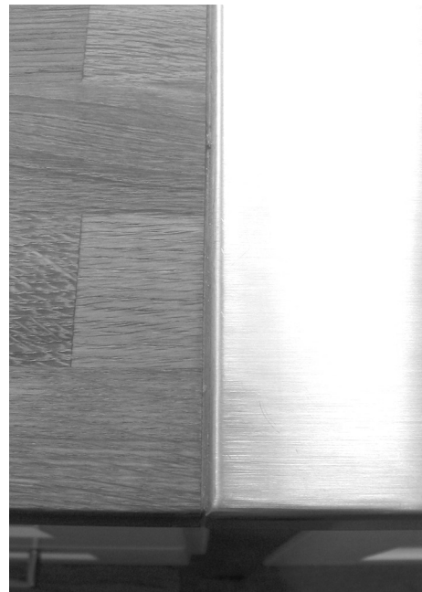
Silicon joint between wooden worktop and adjacent stainless steel sink unit.
