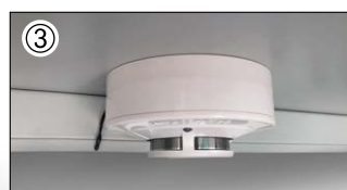
Smoke detector and temperature sensor
