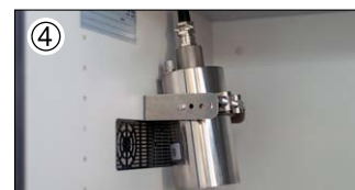
Warning/fire suppression system
