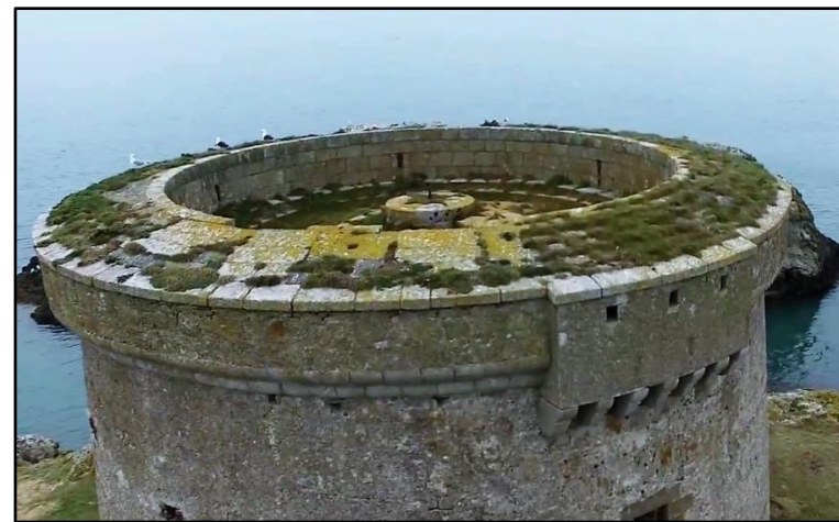
Plate 18 View of tower roof from Drone footage (courtesy of Ken Doyle, Ireland's Eye Ferries)
