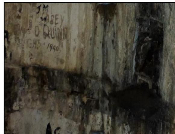
Plate 16 Interior of tower, showing graffiti above original floor level
