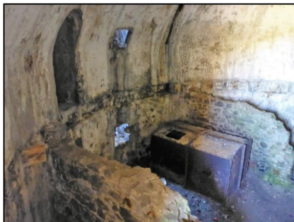
Plate 15 View of interior of tower, showing metal trunk and walls dividing undercroft
