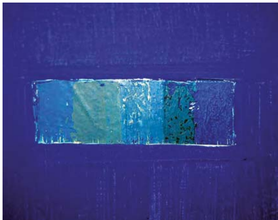
Fig. 1: Villa La Roche, passage from main hall to maid's room. Paint layers visible after restorator Ariel Bertrand laid open the paint layers. The colors range from a medium ultramarine blue shade on the left (a blue acrylic paint from 2001) to the sample on the right, which is the original ultramarine blue in glue paint fixed with casein and deepened with bone black in 1925-1926. What causes such differences, how do they affect architecture?
