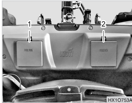
(1) Fuse Box 1 (2) Fuse Box 2
