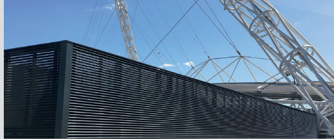
Wembley Stadium, London. Product 1UL/SH screening louvre.
