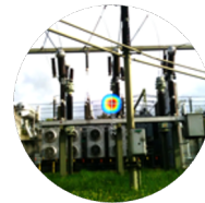
Detection of partial discharge
