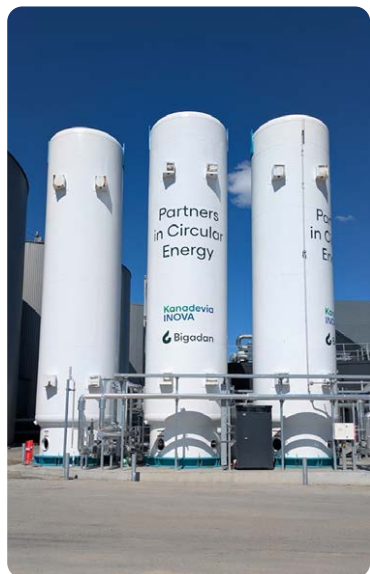
A new CO 2 liquefaction facility built by Kanadevia Inova in Kalundborg, Denmark
