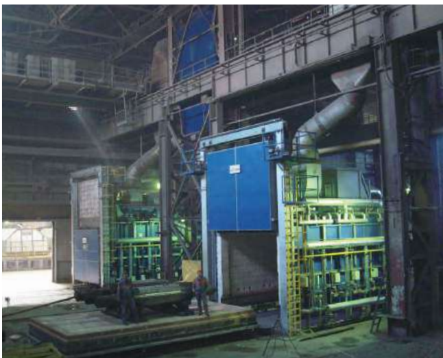
gas heated furnaces - 70 m 3 - 1150°C
