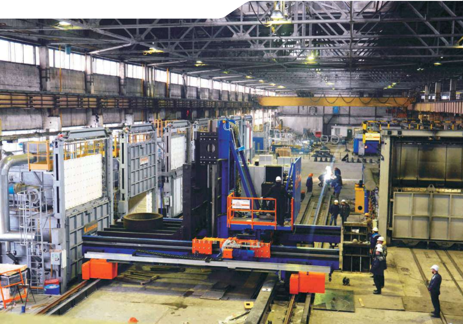
furnace line with quenching tanks and manipulator
