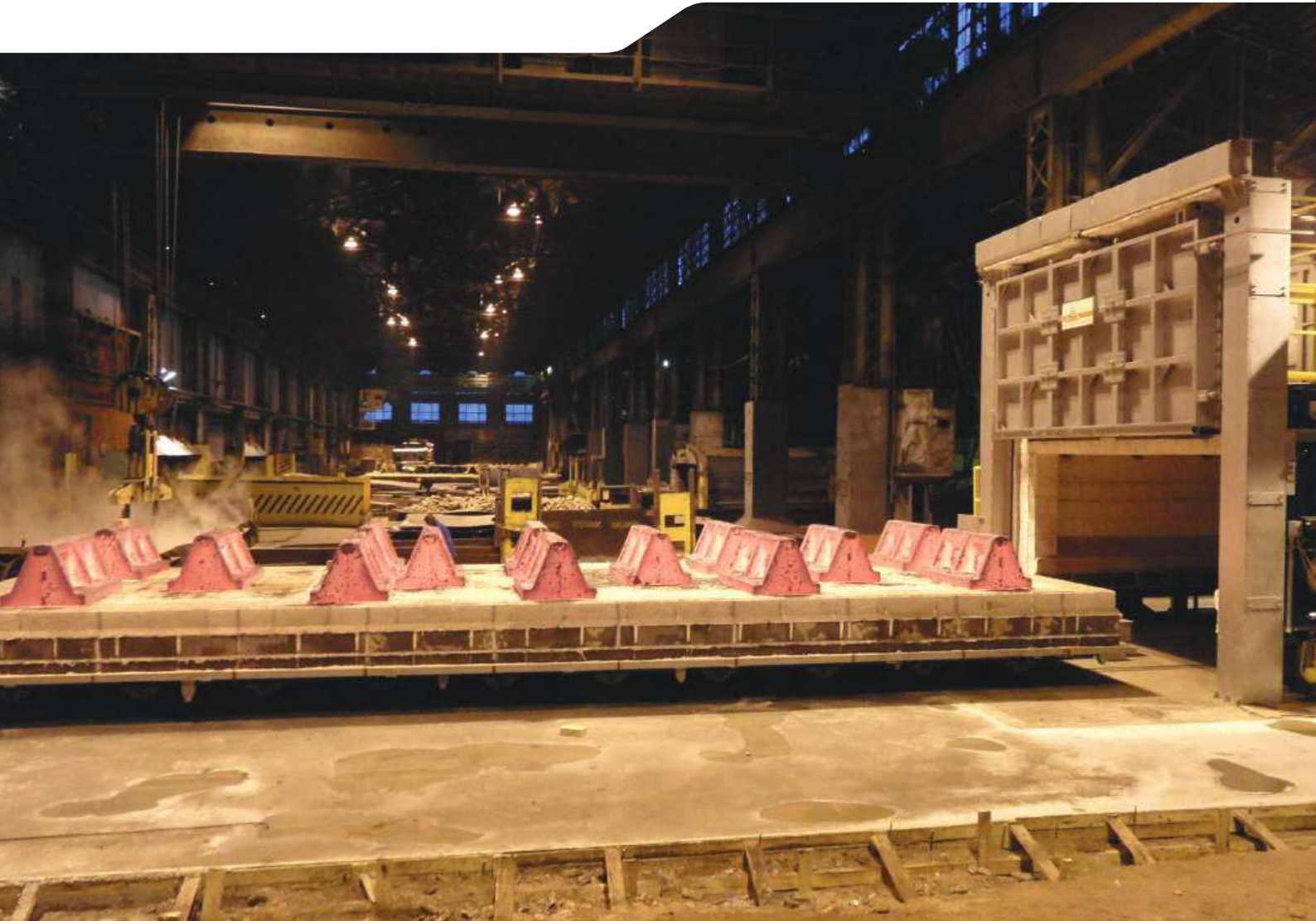
gas heated furnace - 51 m 3 - 1200°C
