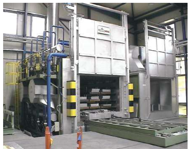
gas heated furnace & cooling chamber - 20 m 3 450°C
