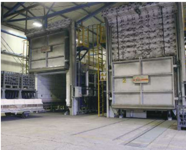
gas heated furnaces - 6 m 3 - 1100°C
