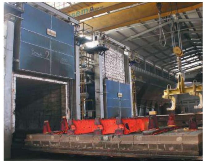
gas heated furnace - 70 m 3 - 1150°C
