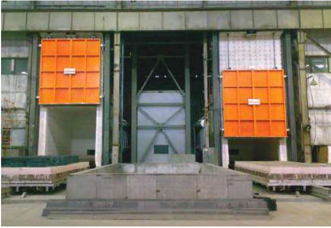
gas heated furnaces with quench tank - 59 m 3 -
