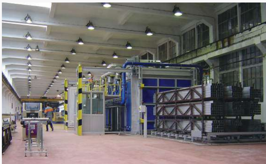
gas heated aging oven - 12 tons - 250°C
