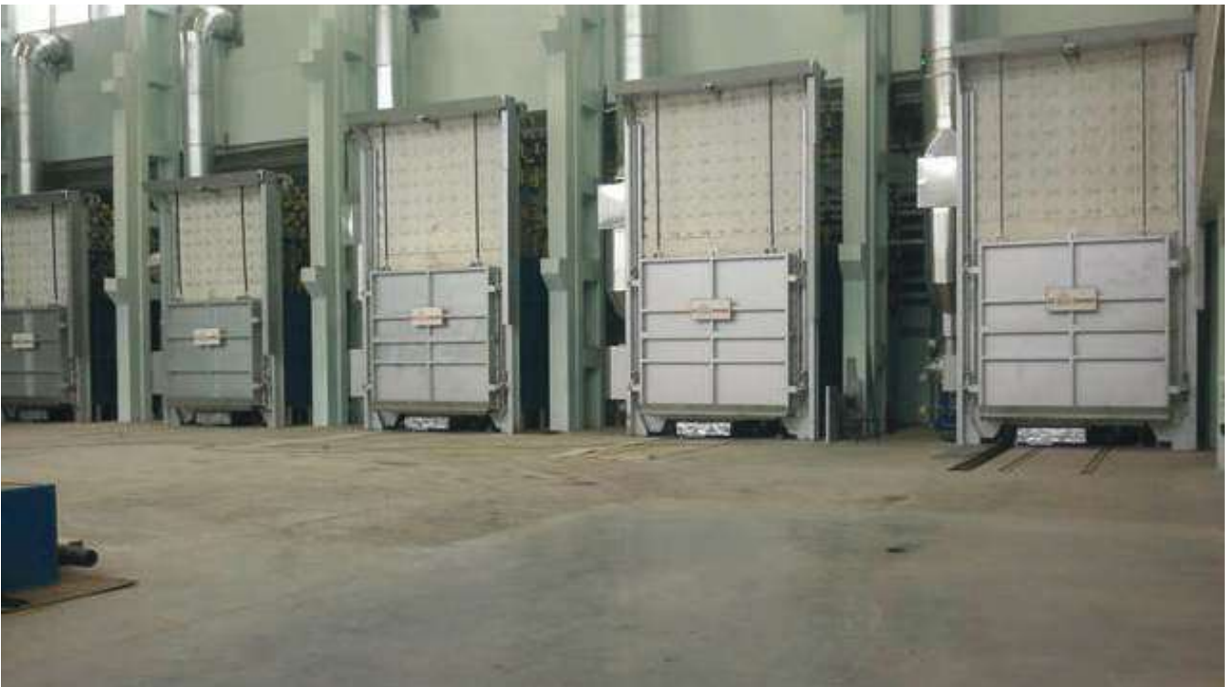
gas heated furnaces - 6 m 3 - 1300°C
