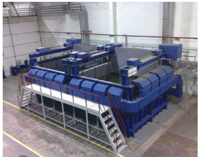
quench tanks with lifting table - water/oil - 100 m 3
