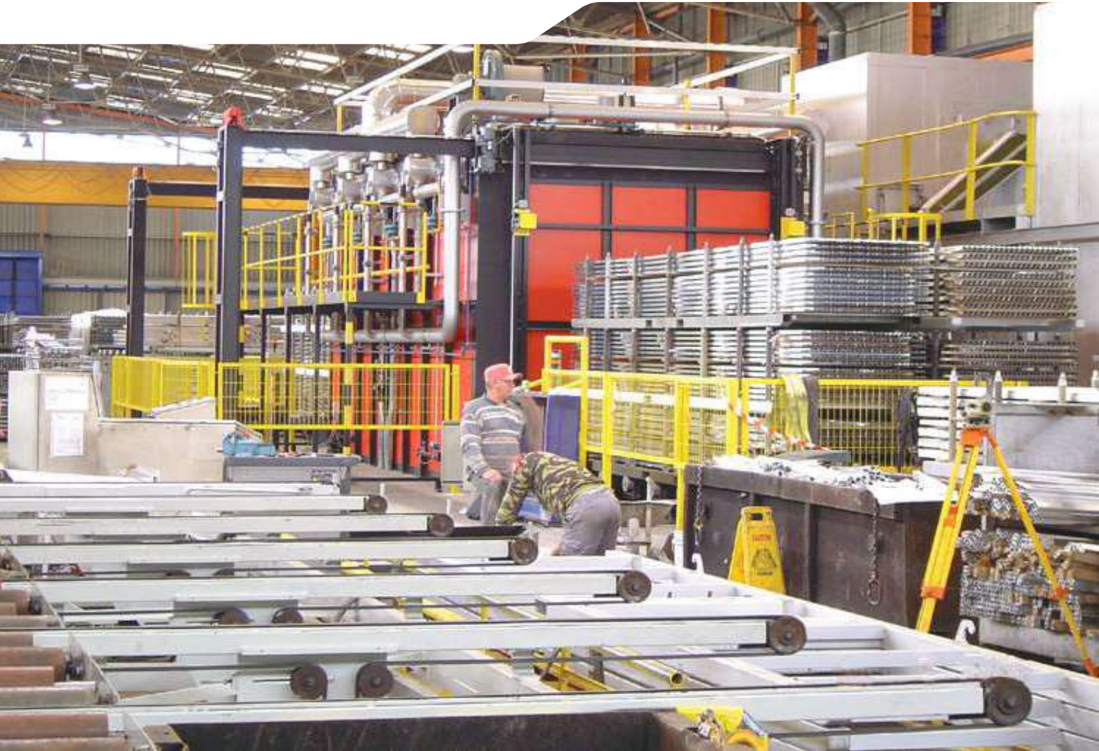
gas heated aging oven - 15 tons - 250°C
