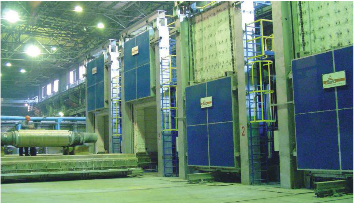
gas heated furnaces - 34 m 3 - 1200°C
