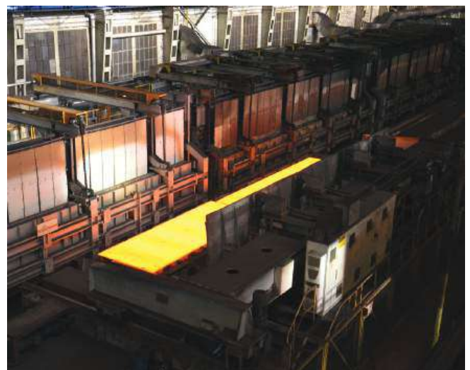
gas heated reheating furnace line with manipulator - 15 m 3 - 1.200°C
