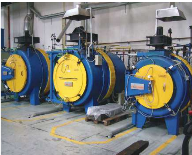
electro heated furnaces with controlled atmosphere (N 2 , H 2 , NH 3 , CO 2 ) & rapid cooling- 3 m 3 - 650°C
