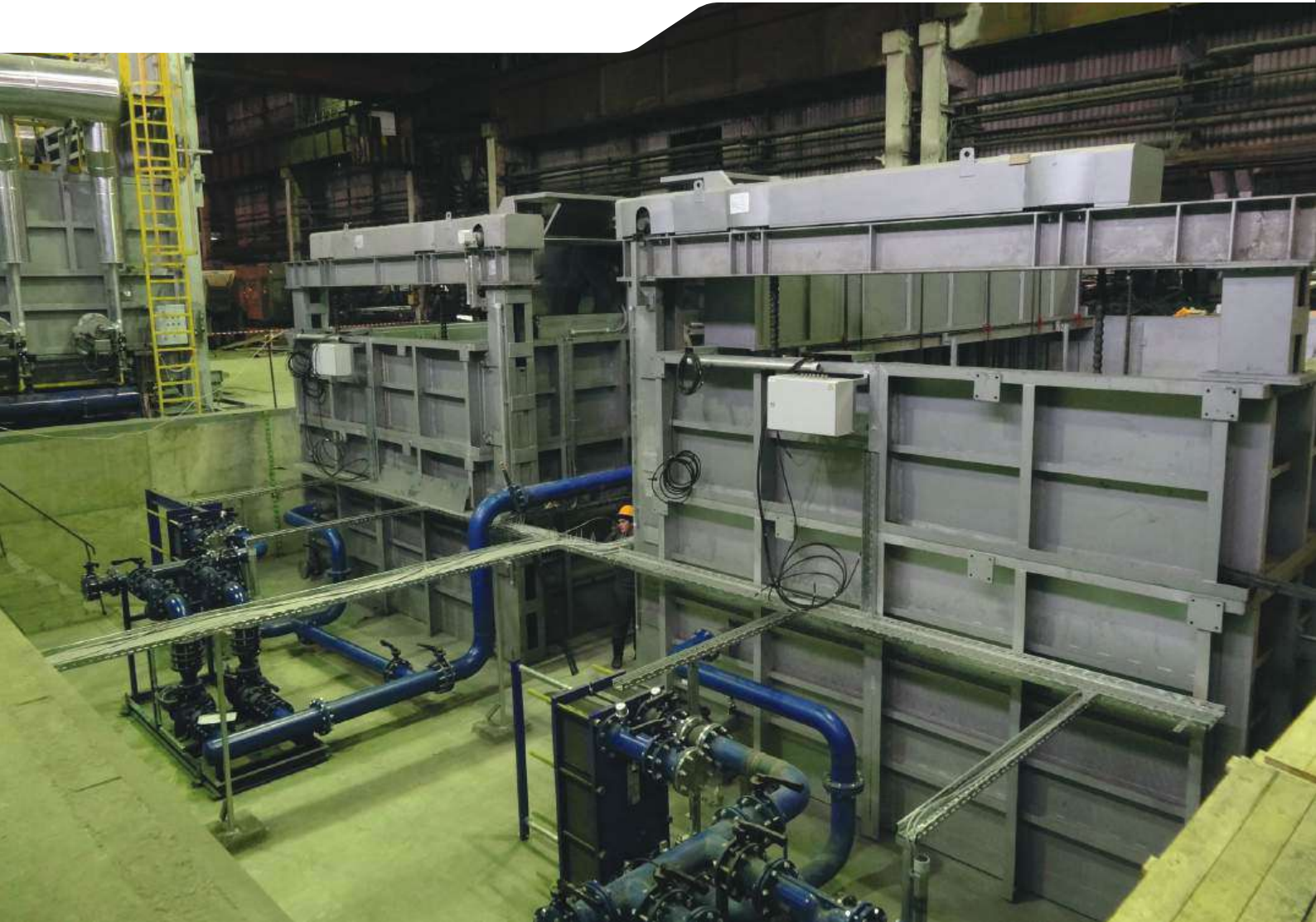
quench tanks with lifting table - water/polymer - 100 m 3
