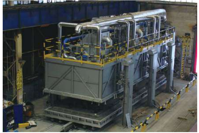
gas heated furnace - N 2 /natural gas atmosphere - 22 m 3 - 950°C
