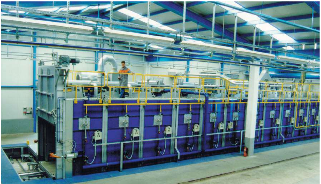
gas heated kiln car conveyor furnace - 28 m - 250°C
