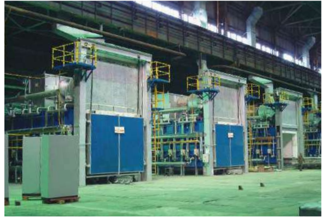
gas heated furnaces - 47 m 3 - 1100°C
