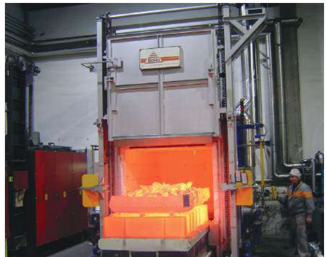
gas heated furnace - 3 m 3 - 1100°C
