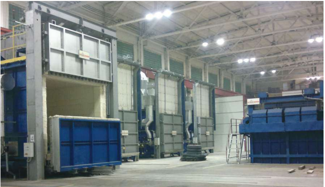
gas heated furnace - 50 m 3 - 1300°C
