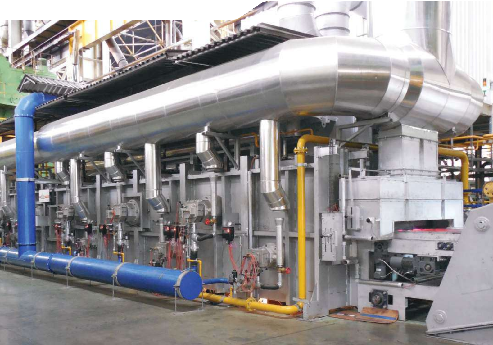
gas heated step chain conveyor furnace - 950°C
