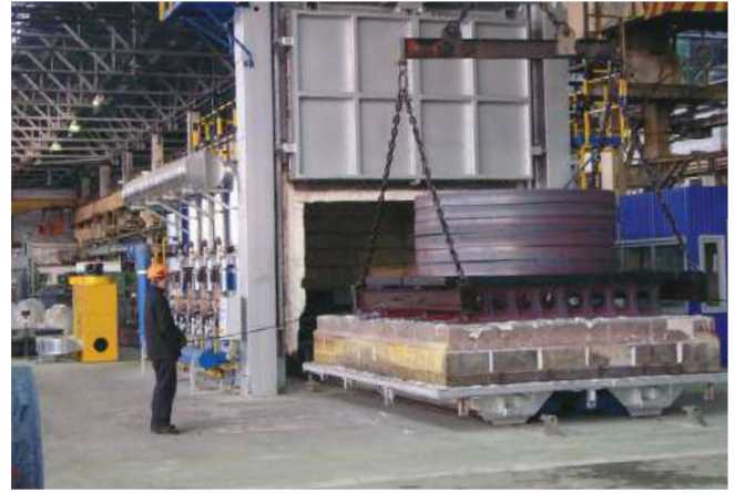
gas heated furnace - 16 m 3 - 1100°C
