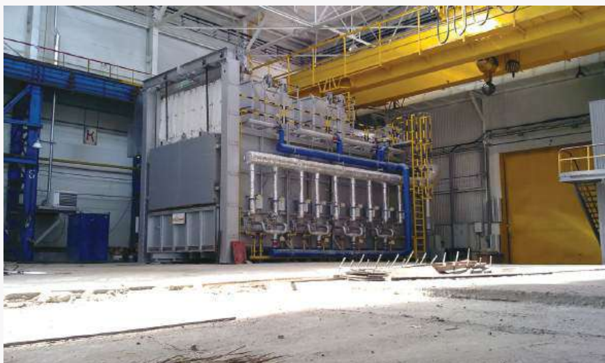
gas heated furnace - 90 m 3 - 1150°C
