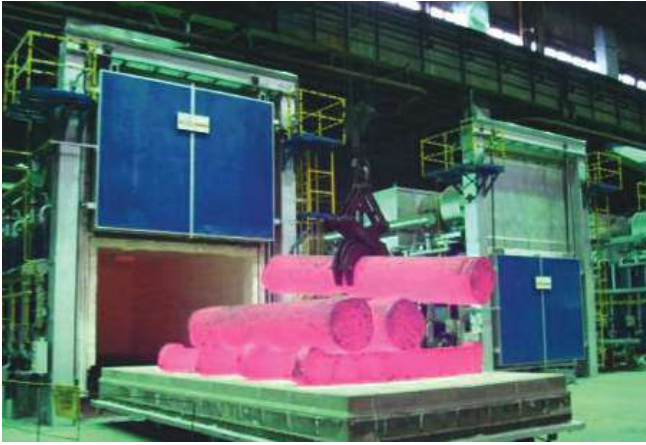
gas heated furnace - 55 m 3 - 450°C
