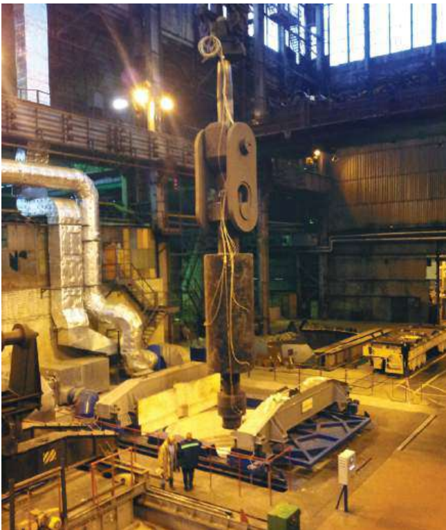
electro heated pit furnace - 175 tons - 22 m load - 1100°C
