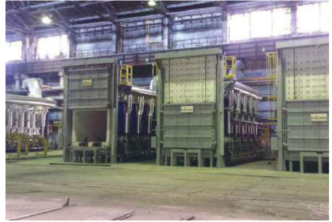
gas heated furnaces – 23 m 3 – 1000°C
