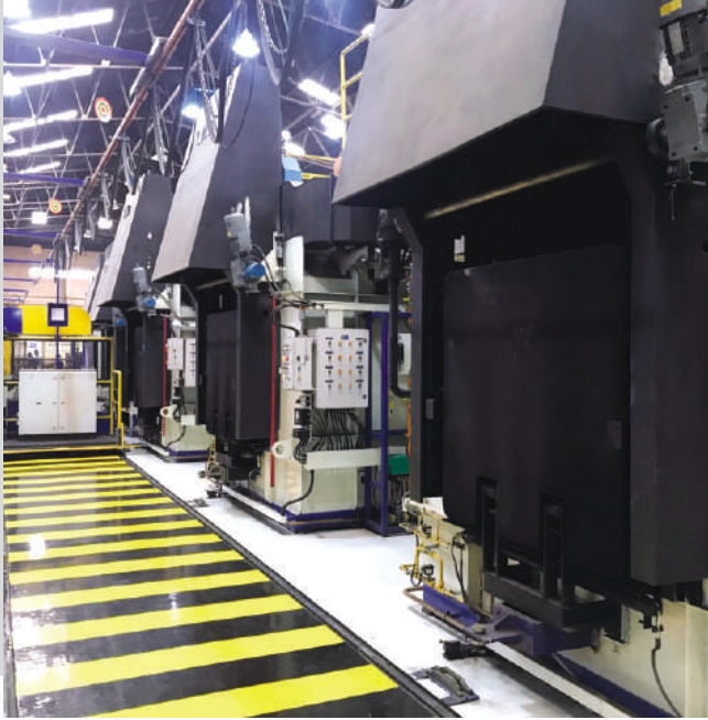
Charge Loading Side
