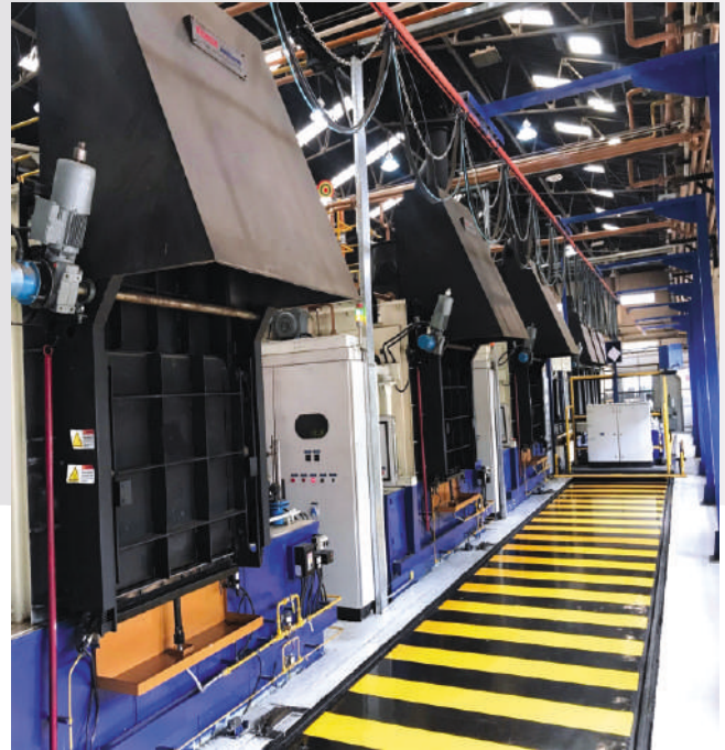
Charge Unloading Side
