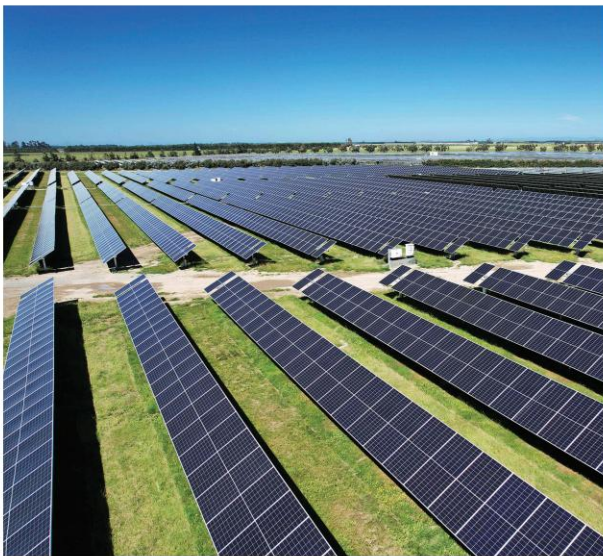
Lauriston solar farm
