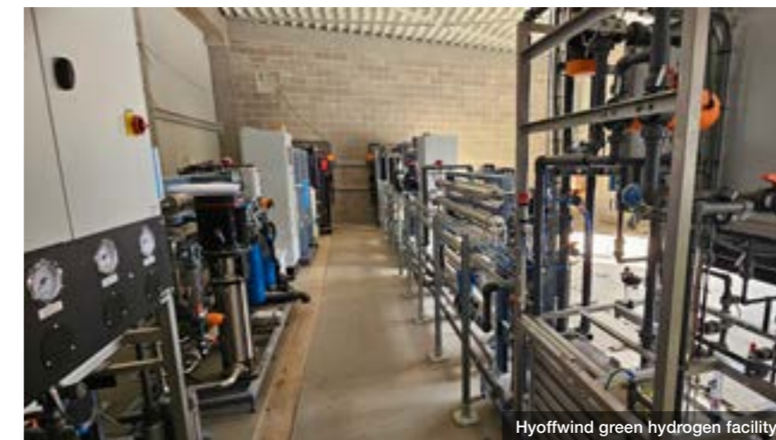
Hyoffwind green hydrogen facility
