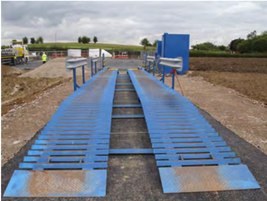
Plate 3.14: Vehicle wheel wash facility
