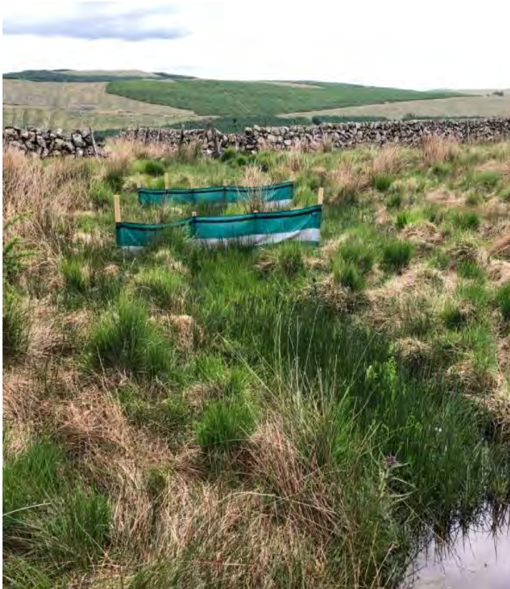
Plate 3.4: Typical silt fencing
