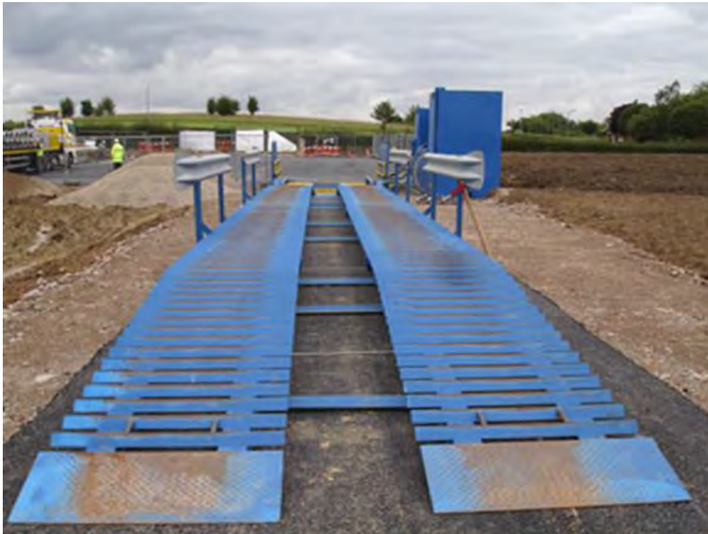
Plate 3.14: Vehicle wheel wash facility
