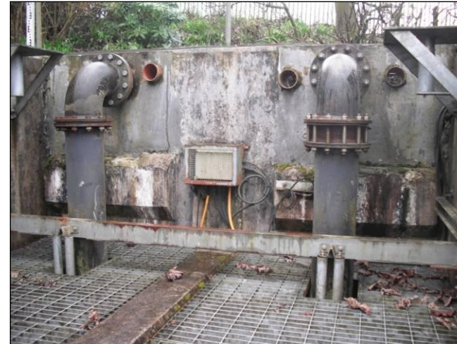
Figure 11: Molendinar Pumping Station
