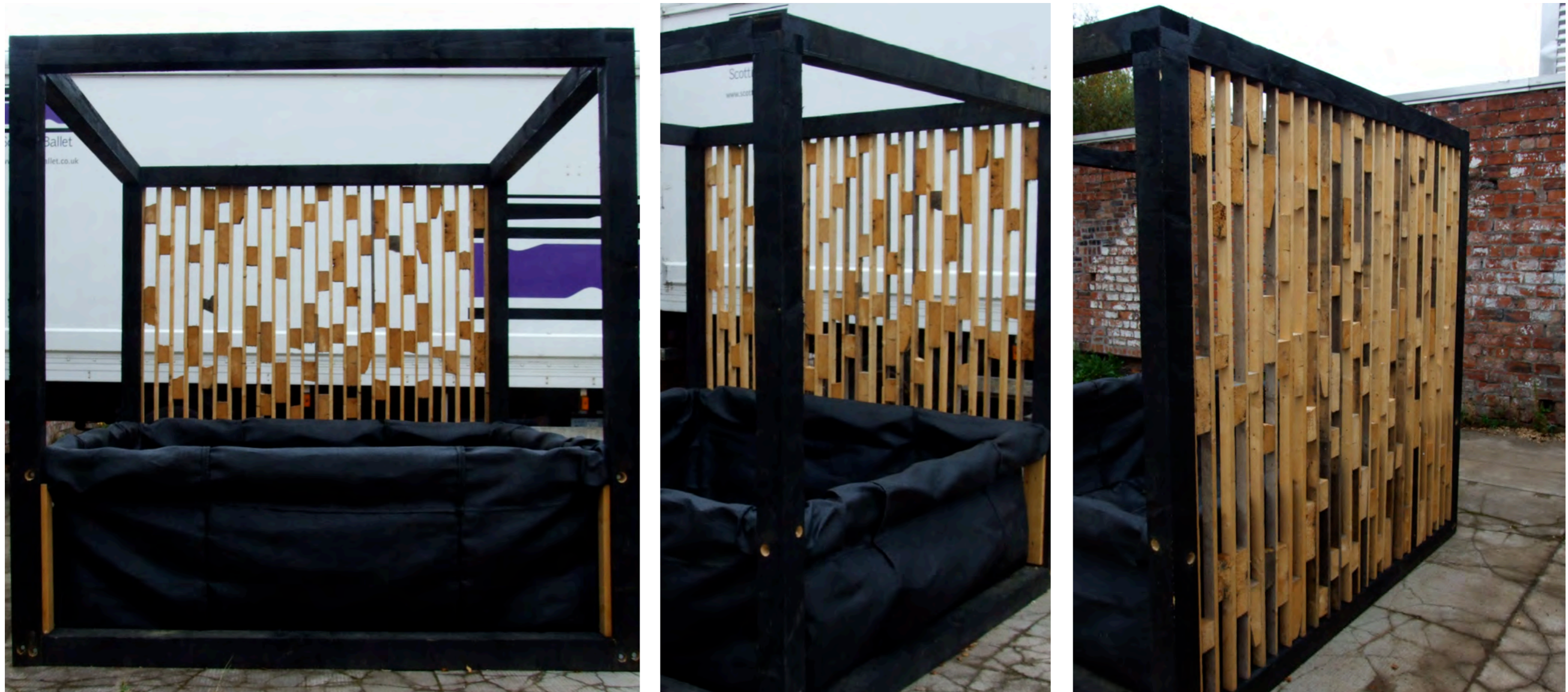
Proto-type perimeter raised planter with screen - under construction. The screen is fabricated of waste palette wood and scaffolding boards.
