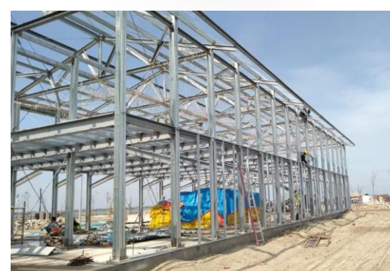
Patimban Port Office, Subang is using LYSAGHT® Cee Purlins as main structure for Pre-Engineered Building System
