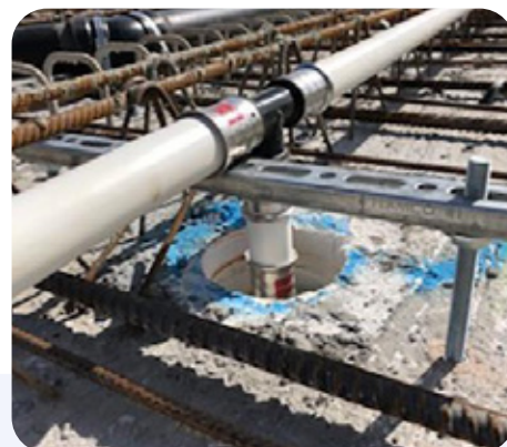
Not embedded 50P's mounted at the building site
