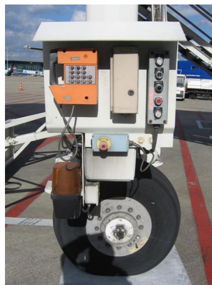
Fig. 50. Locatie externe noodstop boarding bridge pier B
