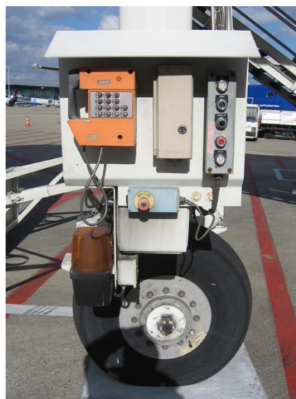
Fig. 49. Locatie externe noodstop boarding bridge pier B
