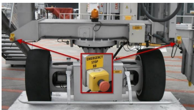
Fig. 48. Locatie externe noodstop boarding bridge pier A
