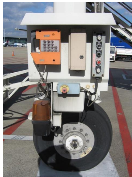
Fig. 49. Locatie externe noodstop boarding bridge pier B
