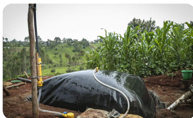
A Sistema.bio prefab biodigester installed in Kenya. Copyright Sistema.bio
