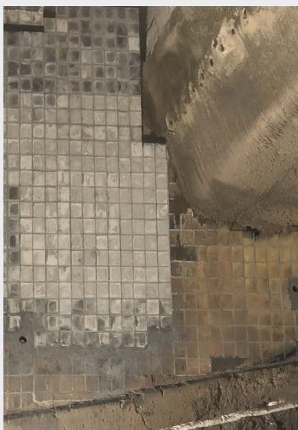
Application in waste-to-energy boiler
