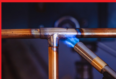
Cyclone Flame Burner
