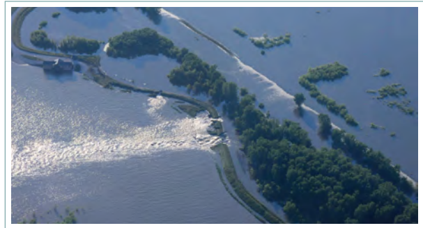
Mississippi River levee break. Photo: Joceyln Augustino/FEMA
