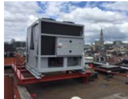
Air Conditioning Building Brussels, Belgium
