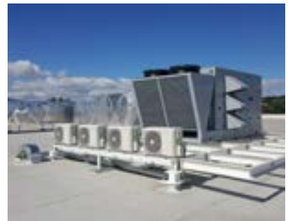
Aki Chaves, Portugal - 2 Roof Top SysAer 120 H
