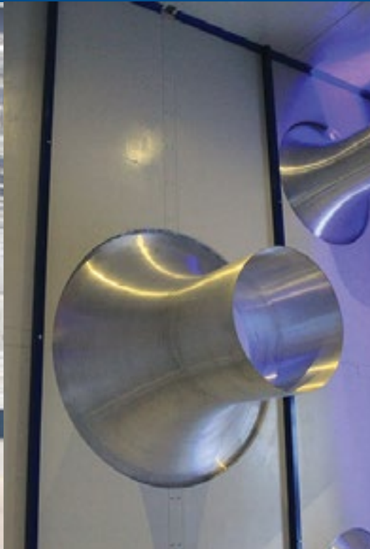
Air Flow Chamber, India.
