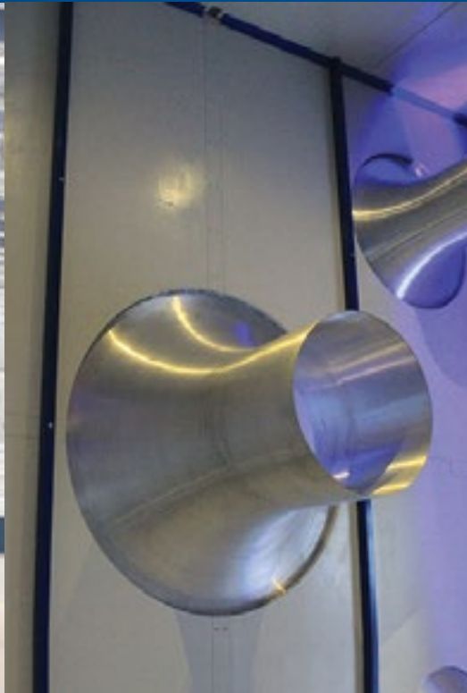
Air Flow Chamber, India.
